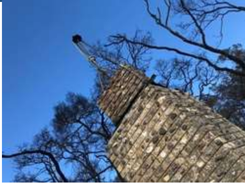
Chimney antenna stand and rotor after the fire. (photo KU6J)
